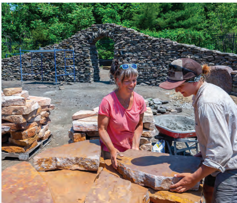
Lifting a sandstone slab, Thea Alvin, left, works with her crew and Rowan students to build the sculpture just east of Discovery Hall.
